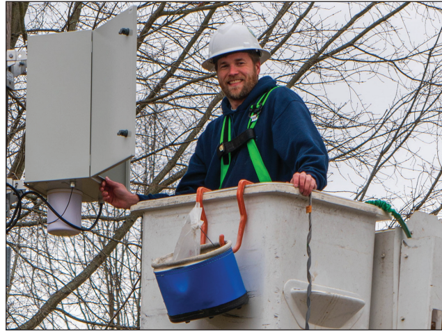
Wesley Cox, Fiber Installation/Repair Technician 2, installs a free, public WiFi hotspot at the Davy Crockett Cabin in Rutherford, Tenn.
