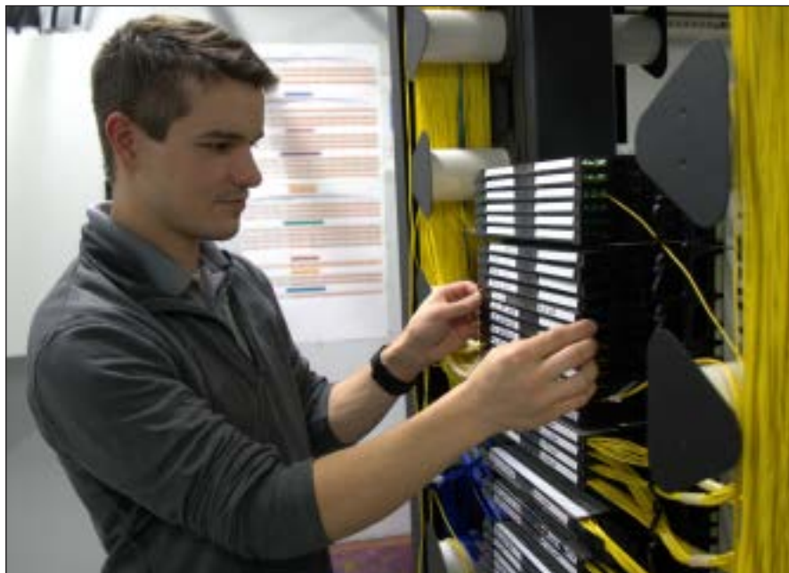
Network Technician Taylor Coomer connects a GPON (Gigabit Passive Optical Network) circuit. Doing this completes the high-speed fiber connection to our members' homes. Like Gibson Electric, our Gibson Connect team is made up of local, dedicated folks who truly care.
